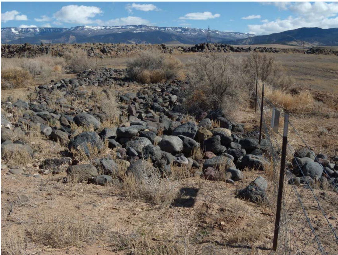
GRJ 3/2011. PL-4. Riprap erosion protection near the southeast corner of the perimeter fence.
