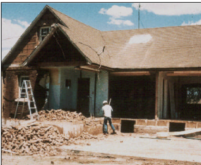
The Harry Randall house in Monticello was one of the first properties to be remediated.
