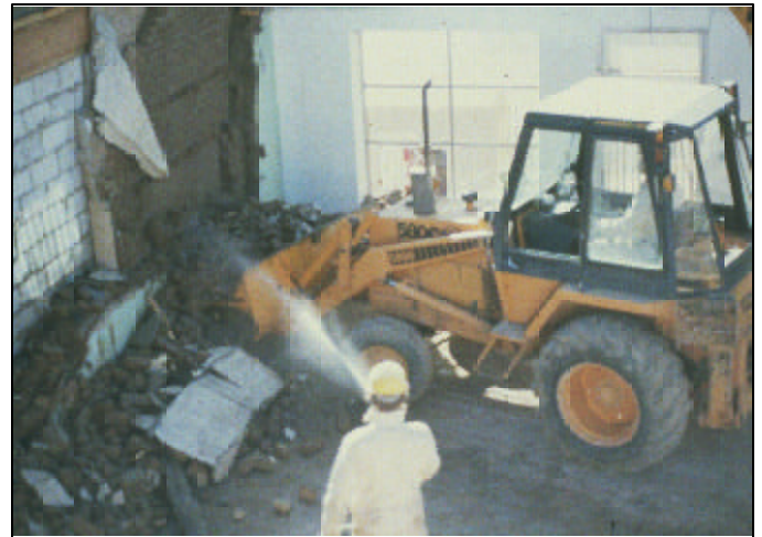
Contaminated materials required the use of heavy equipment for remediation of the Montgomery Ward store in Monticello.
